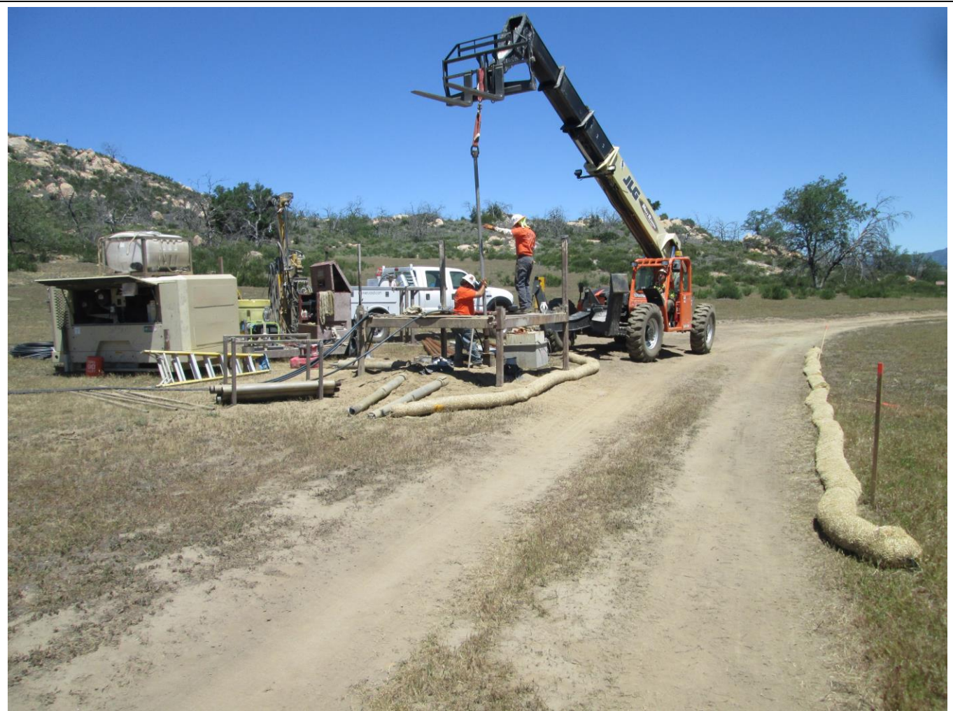
Photo 2: Micropile construction crews were observed drilling, setting bar (pictured), and grouting during this reporting period. Straw wattle BMPs were installed around project activities at this location in accordance with the project SWPPP.
