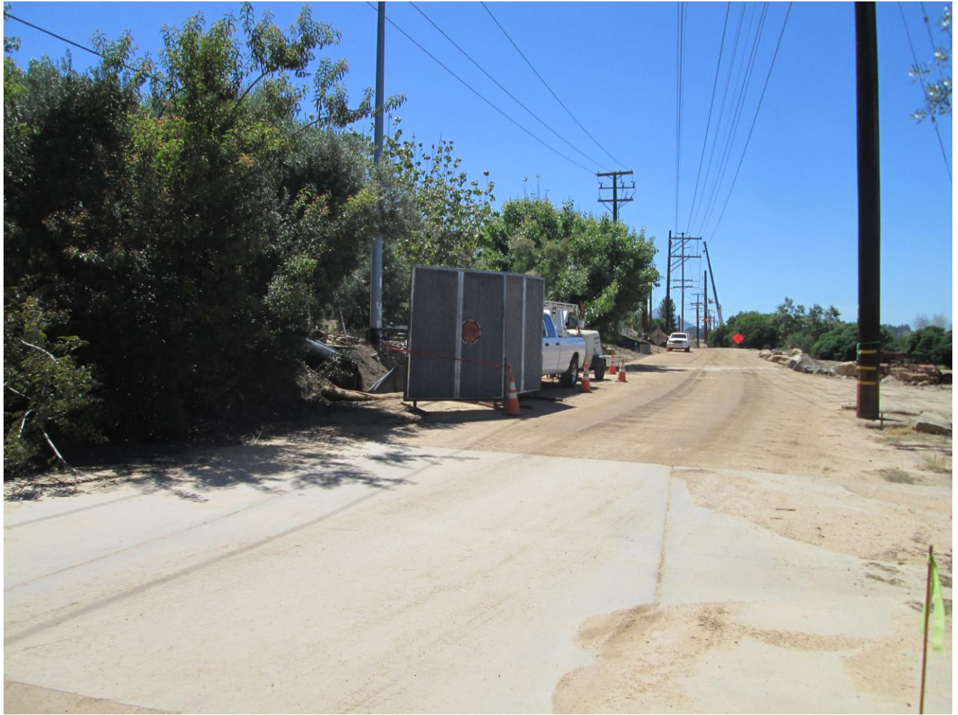
Photo 3: Noise meters and sound barriers were installed during hand digging activities at Location 8 along Creelman Lane in order to ensure that noise limits did not exceed mitigation thresholds and noise was reduced near sensitive receptors (MM NOI-2). Green flagging (bottom right) was installed subsequent to nesting bird surveys in order to ensure crews adhered to buffer requirements around these areas (MM BIO-4).
