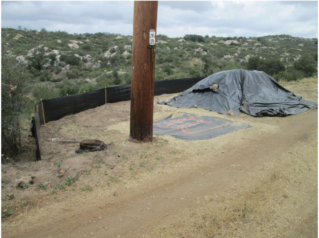
Photo 7: Previously drilled pole holes were covered to prevent wildlife entrapment in accordance with MM BIO-3. Stockpiles were observed covered with visqueen and silt fencing used for sediment control was found installed and in good condition in accordance with the Project SWPPP (APM-HYD-1).
