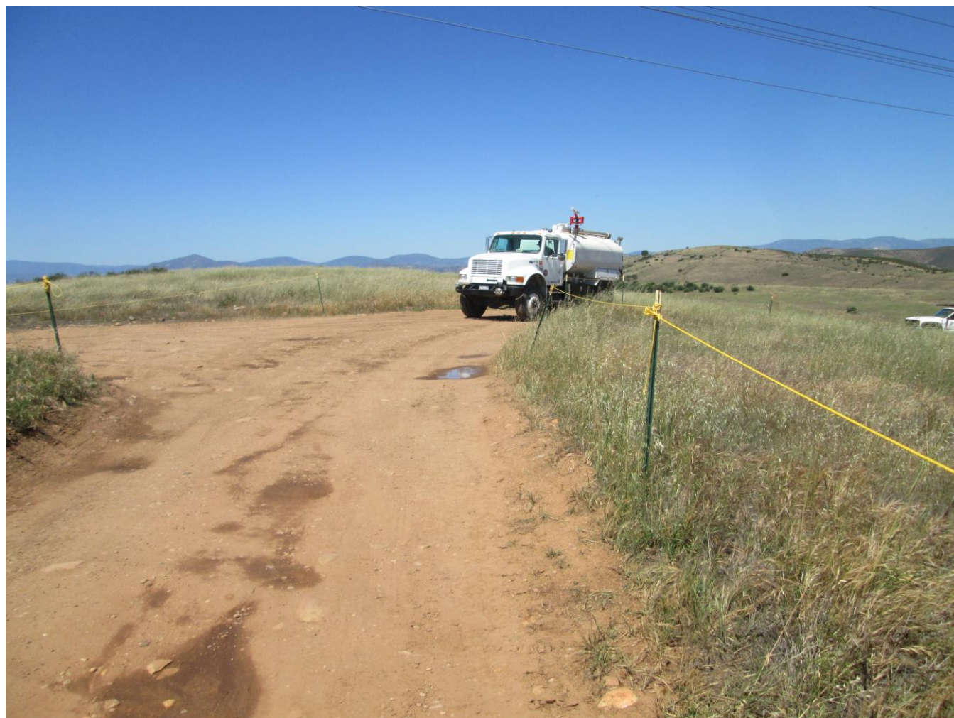
Photo 8: Environmentally sensitive areas were observed delineated in the field and roped off for construction personnel avoidance. In accordance with APM CUL-3, archeological monitors were observed monitoring construction activities that occurred near the sensitive resources and crews were observed respecting avoidance buffers.
