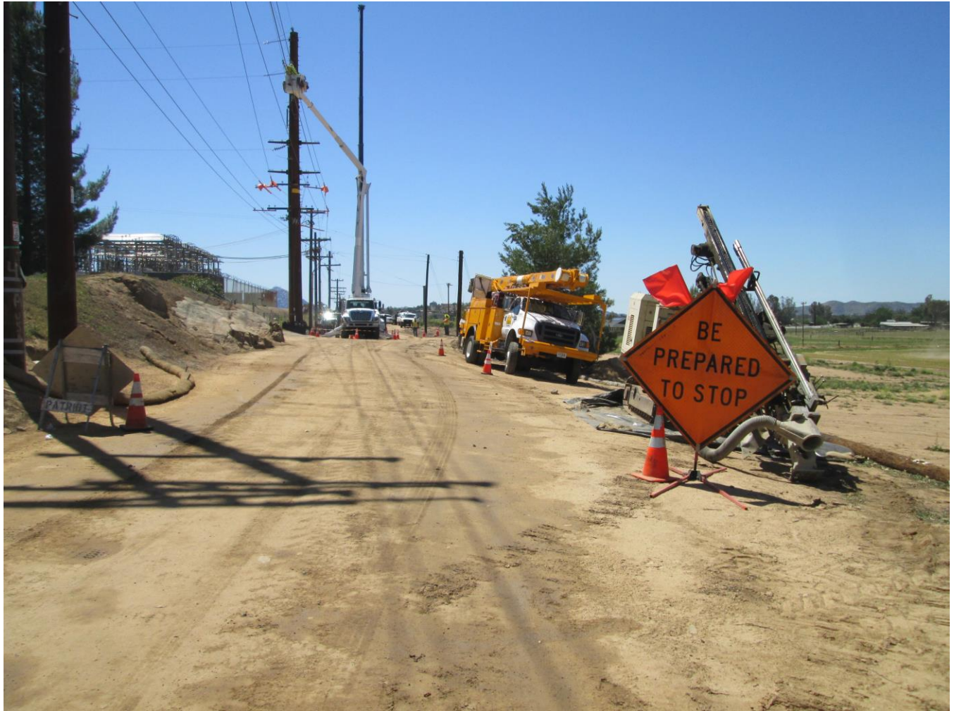
Photo 4: Crews worked to transfer wire onto newly erected steel poles along Creelman Lane. Signage, cones, and traffic personnel were mobilized to direct traffic past pole replacement construction sites in accordance with APM TRA-1.
