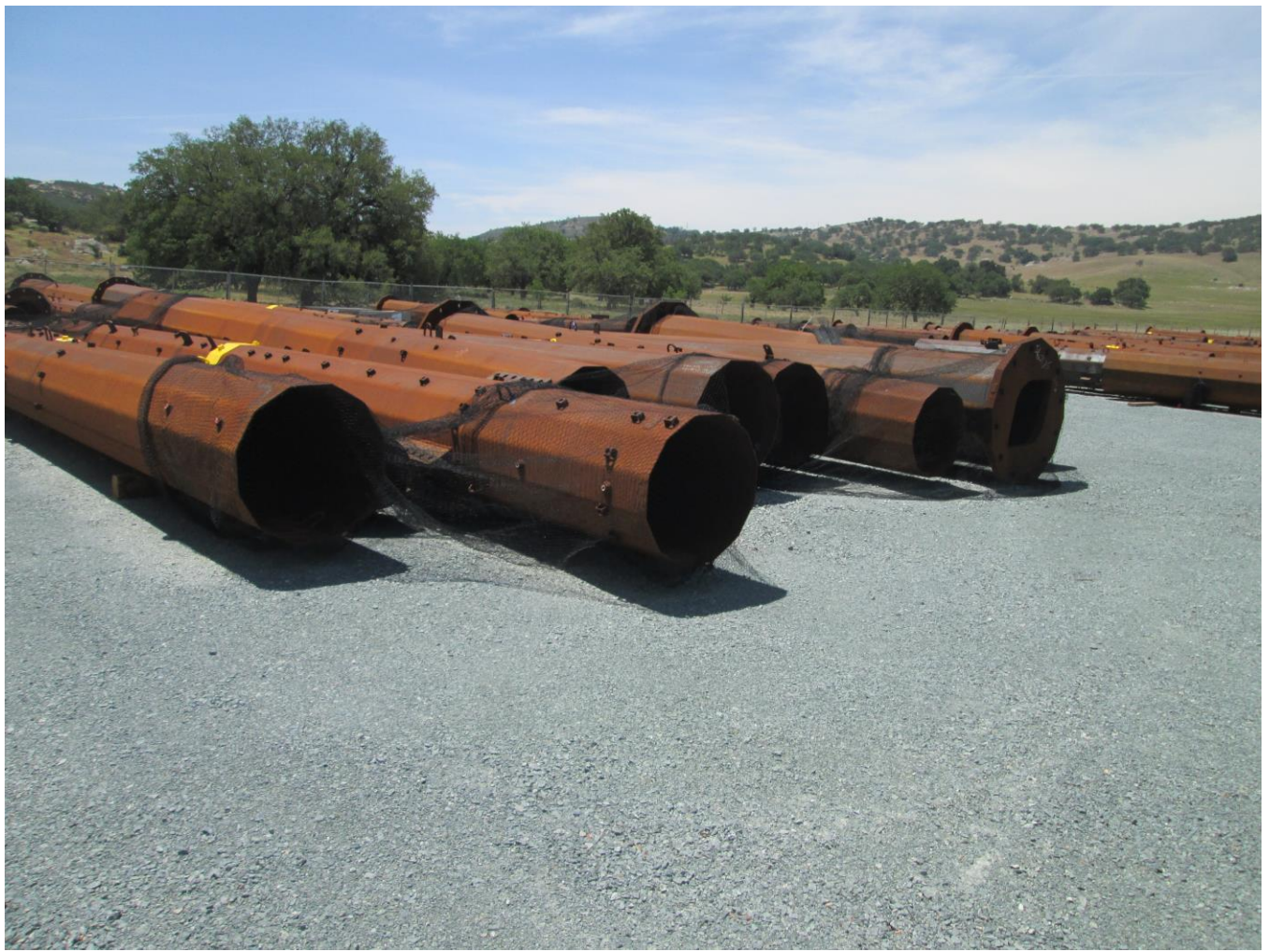
Photo 1: Steel poles were delivered and staged at the Santa Ysabel staging yard. Openings to the poles were covered with nets to prevent wildlife entrapment (MM BIO-3) or prevent bird nesting activities in crevices.
